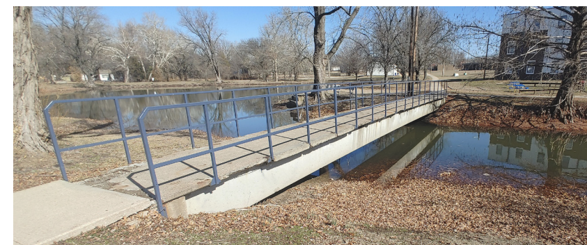
Campus/Academic side of the pedestrian bridge. (Note: deteriorated concrete and exposed rail supports)
